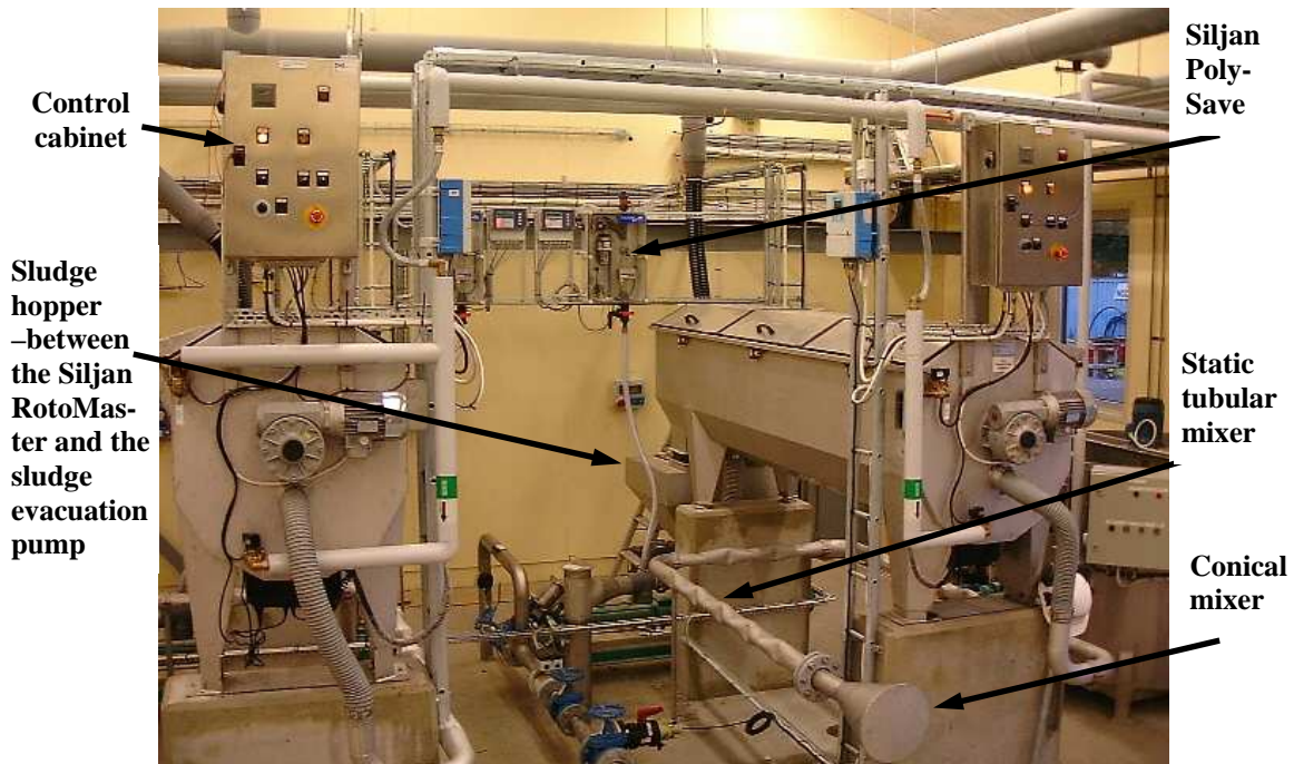
The picture shows 2 pcs. SF 17 Siljan RotoMaster, with auxiliary equipment.
